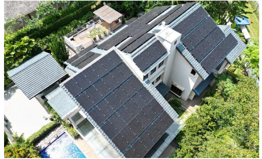
30kWp, Carmen St.
