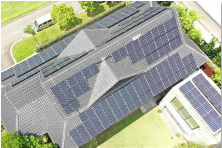
41kWp, Third Avenue
